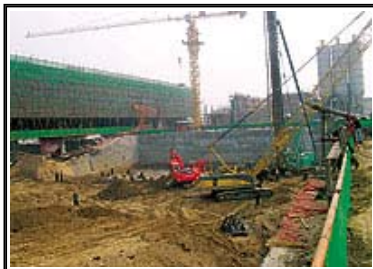
Chinese subcontractor is building the foundations for what will be an eight-story high-security building, but the structure will be built by American crews using all-American materials.
